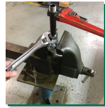
Improper tightening with wrenches
